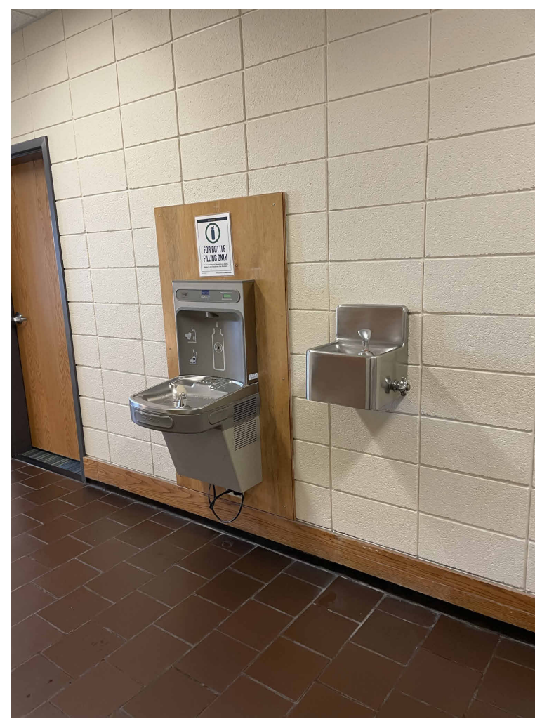
EXISTING FIRST FLOOR DRINKING FOUNTAINS INSTALLED IN EXISTING BLOCK WALL
